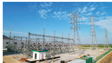
AMATA POWER SUBSTATION 1
